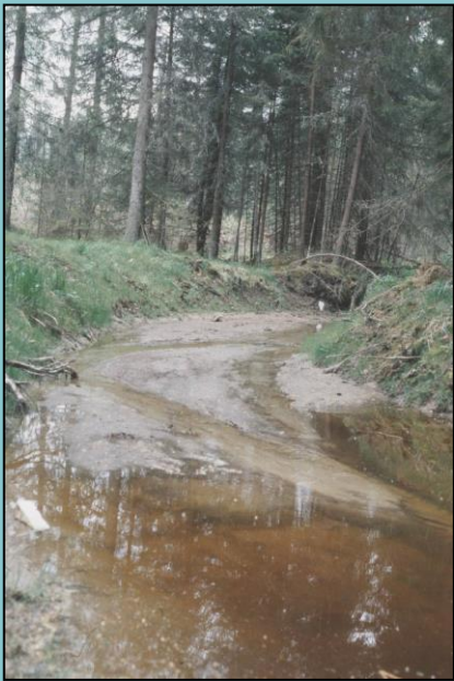
Eroded material settled on ditch bed
